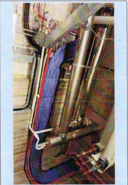
New trap installed at high level.
